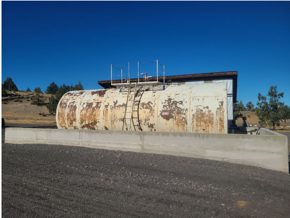
Photograph 3. Large diesel AST within containment.
