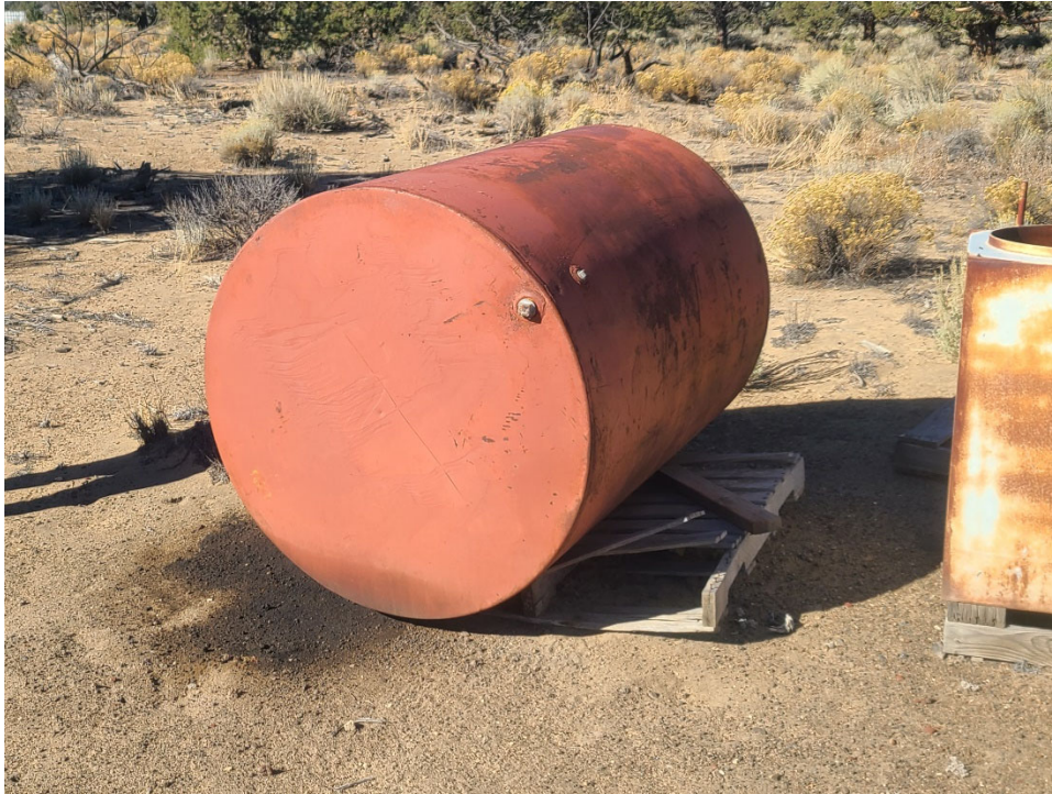
Photograph 5. Oil tank and staining in boneyard.
