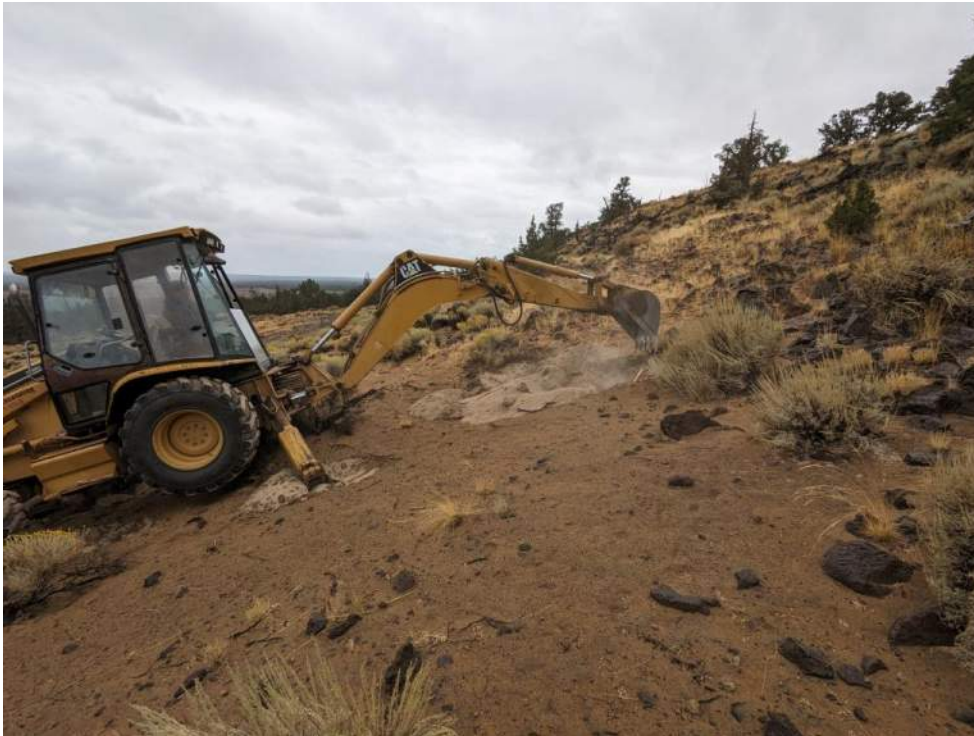
Photo 4. Backhoe excavating into the toe of the slope at the location of TP-4. Sandy colluvium with cobbles and boulders from upslope bedrock.
