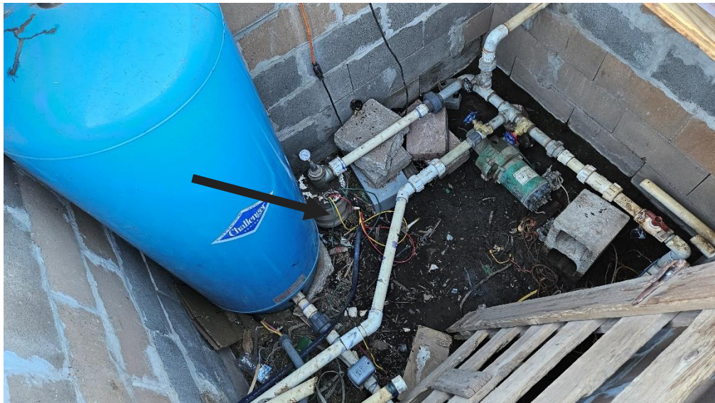
Photo 2. The interior of the water well vault, as seen from the north. The well is shown by arrow.
