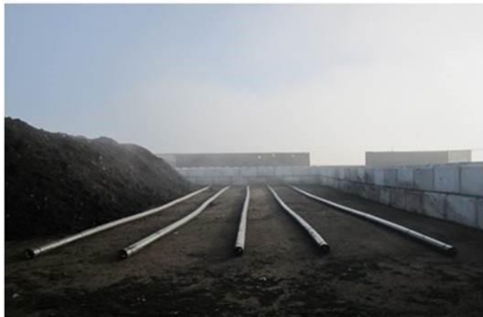
Figure 6-8: Aeration Pipes for Aerated Static Pile Composting
