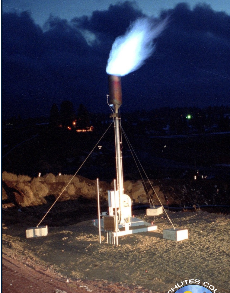
Knott Landfill methane flare, gas collection system built in 2001
